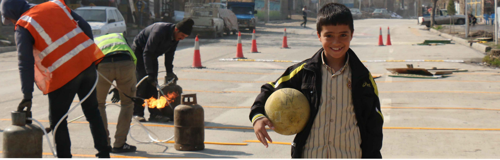
Above: Improvements underway with road markings to delineate and enhance school zone visibility.
