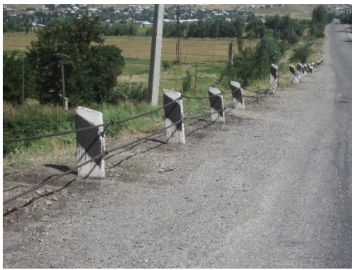
These cables are not tensioned and will not redirect an impacting vehicle. The posts are unforgiving and will lead to significant damage if struck.
