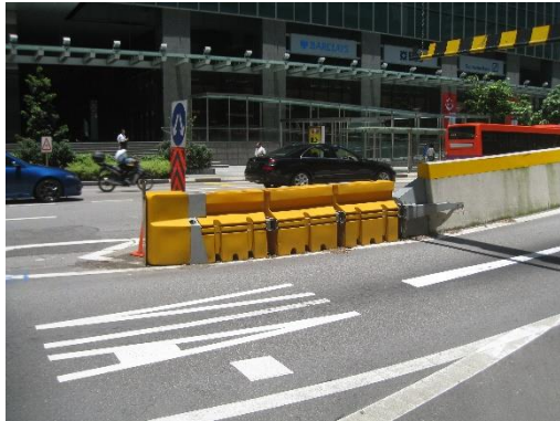
There are several impact attenuators that are approved for use in advance of temporary rigid barrier at work sites
