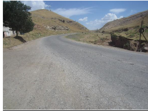
Operating speeds are around 80km/h. Volumes are almost 4000 vpd (total both directions). The highway lacks delineation. Many of the single vehicle crashes have occurred at night.
