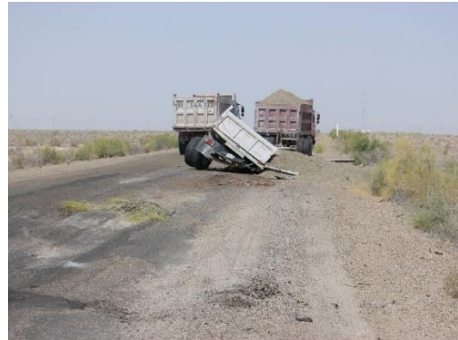
This 55km length of rural highway is to be rehabilitated. It is experiencing many run-off-road crashes
